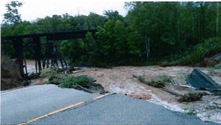
The Trout Brook washout of State HWY 13 near North York/just north of Highbridge July 2016
