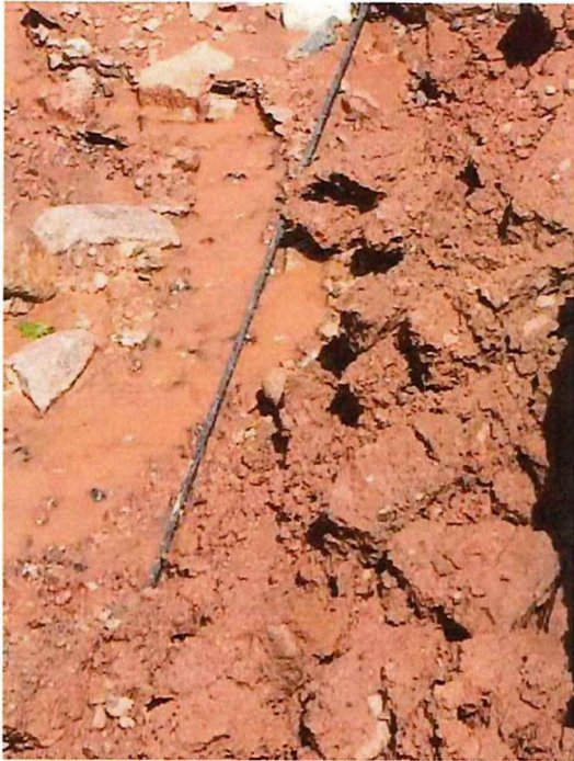
Exposed telephone cable on Poppe Rd. Main cable severed at the Trout Brook washout.
