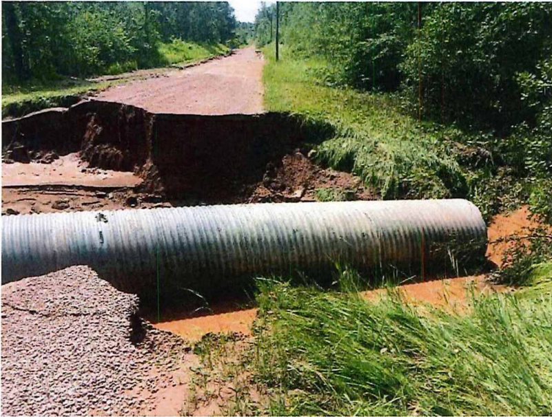
Culvert on Poppe Rd totally exposed after July 2016 Flood. This had been replaced a few years prior as a demonstration model for culverts under a grant from the U.S. Fish and Wildlife, designed by the Federal Engineers.
