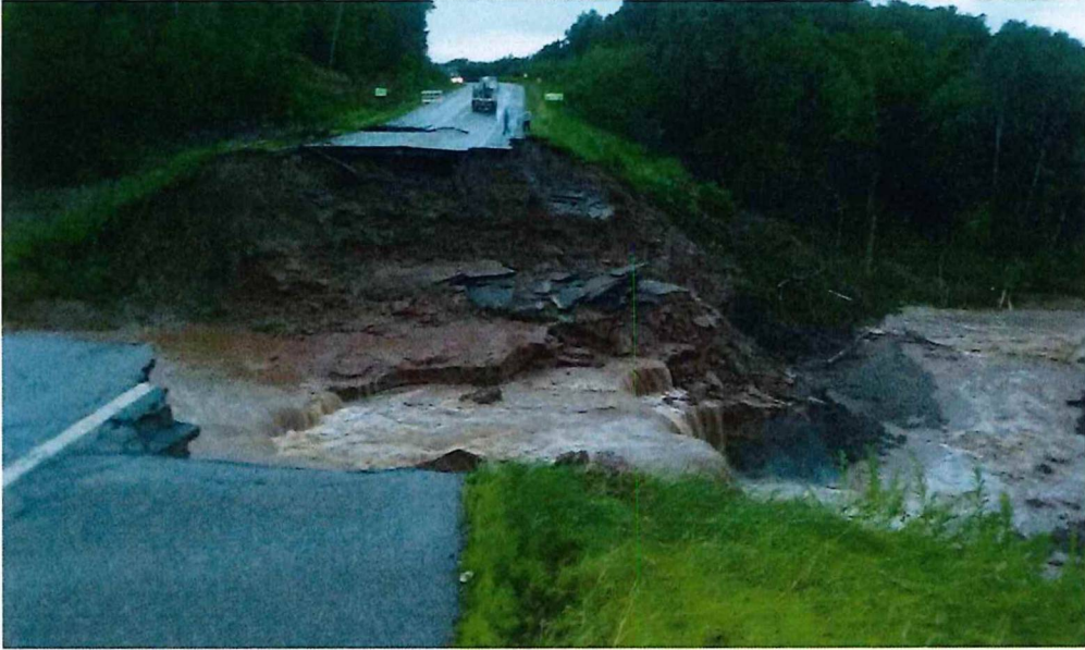
The Silver Creek washout July 2016 of State Hwy 13 just south of Highbridge
