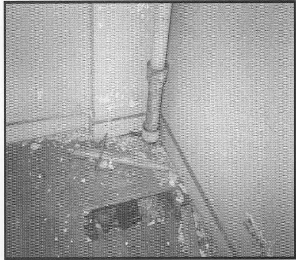
Figure 8.2 Area Should Be Precleaned and Structural Deficiencies in Flooring Repaired Before Lead Hazard Control Begins.
