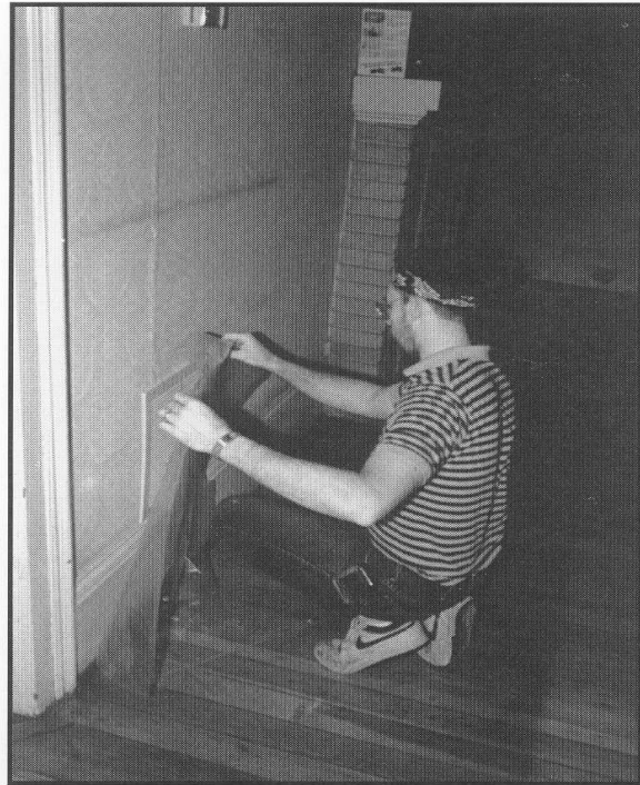
Figure 8.5 Cover the Air Vents With Plastic After Turning Off the HVAC System.
